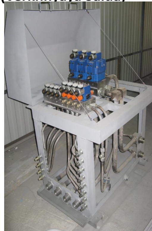
Hydropanel for control of guide valve
