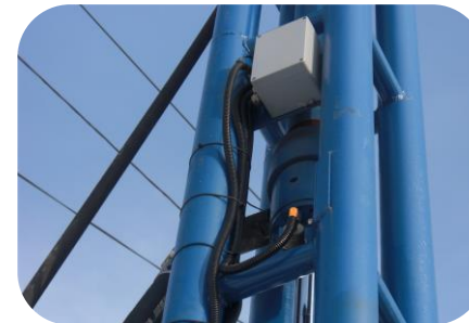
Hydraulic drive (installation) for oil production
