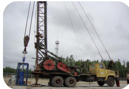
Tests of towers (masts) of load-lifting units
