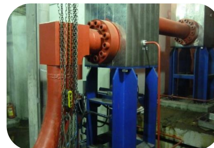
Shut off control and distribution equipment of presses
